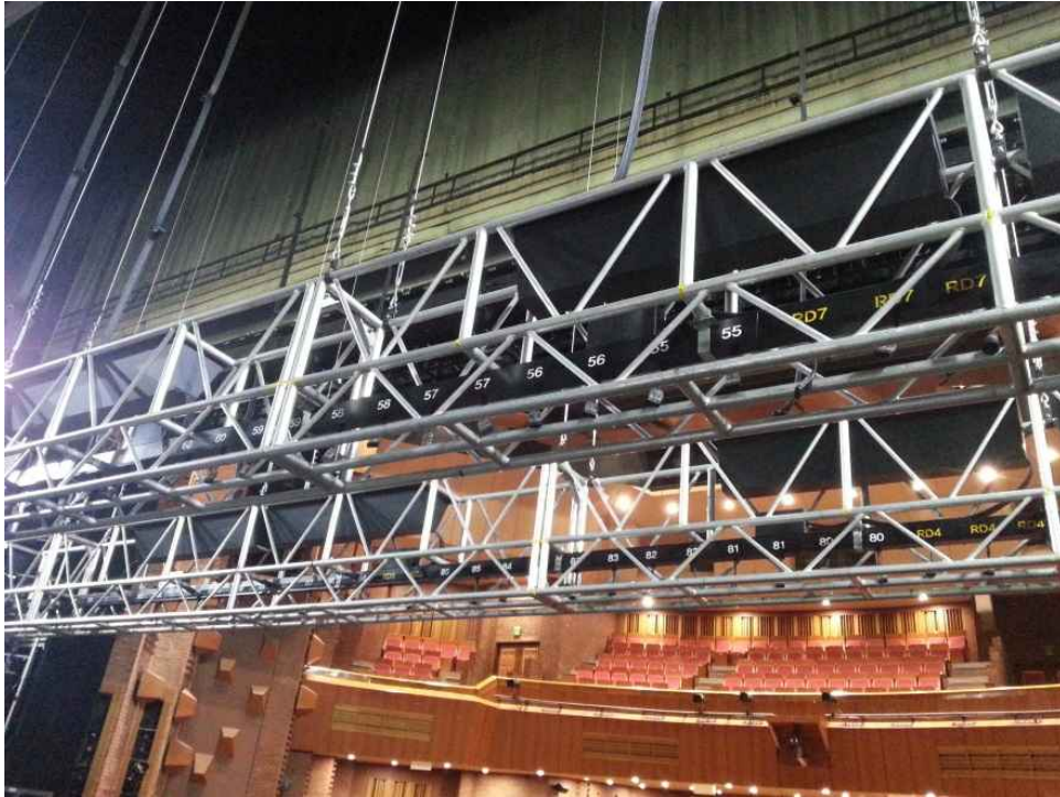
Lighting (Light batten)
