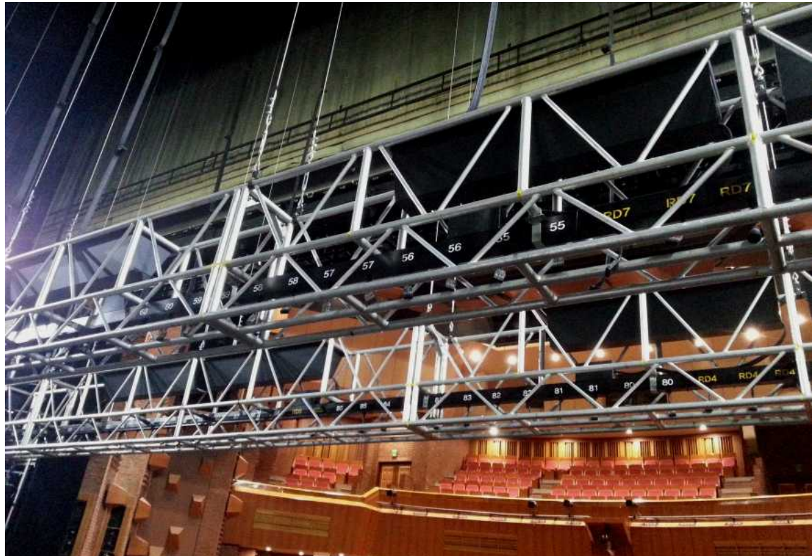
Lighting (Light batten)
