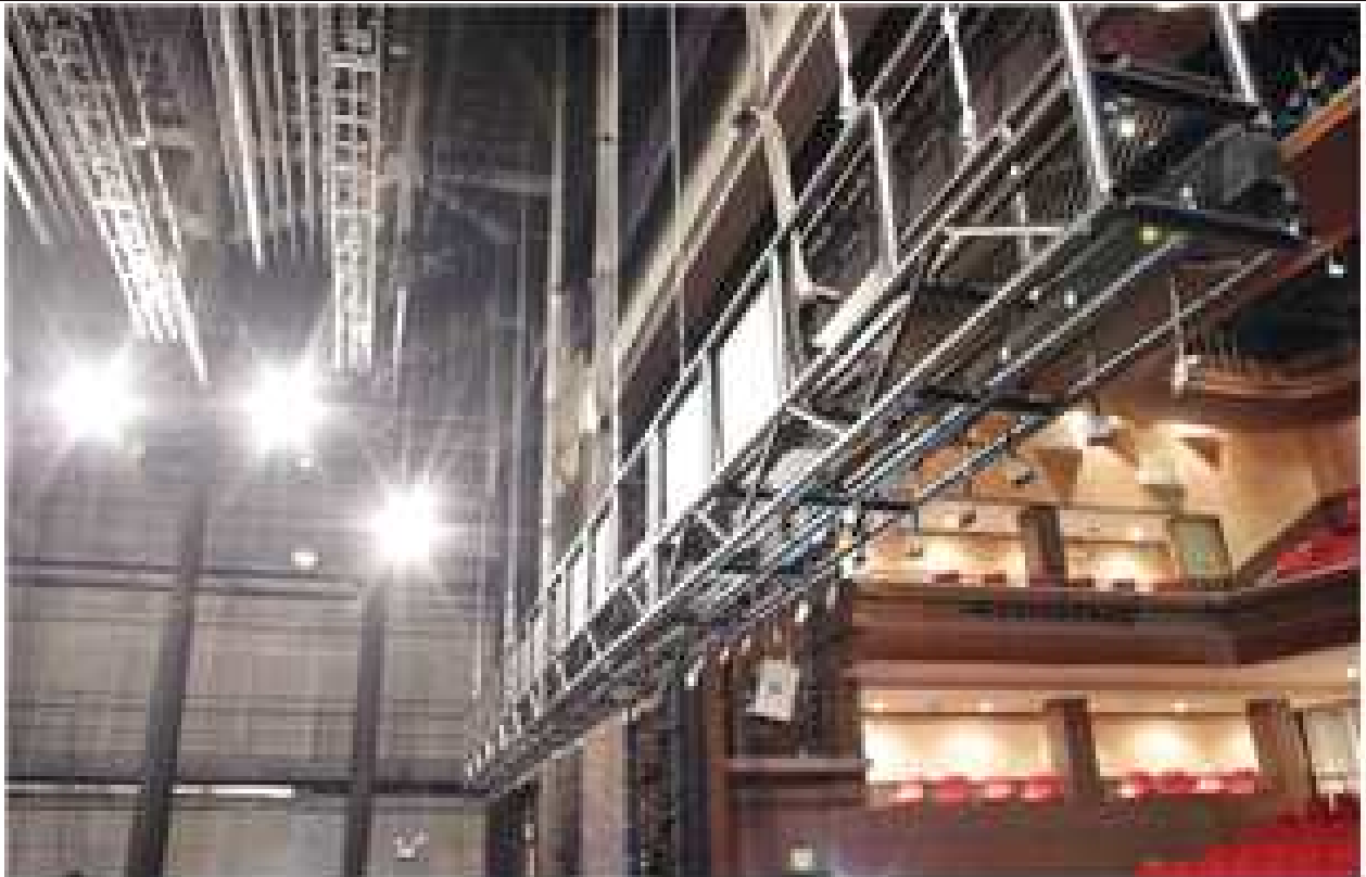
Lighting (Light batten)
